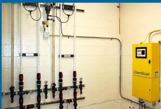
Central Membrane Filters
