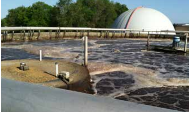
The Alfa Laval SBR's floating decanter and Agri Beef's biogas dome
