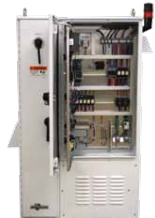
Zone 3: Controls Compartment
