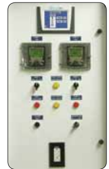
Zone 3: Inner Door of Controls Compartment
