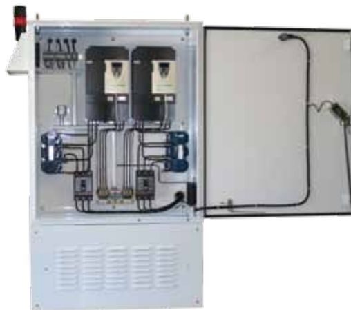
Zone 2: MCC Compartment
